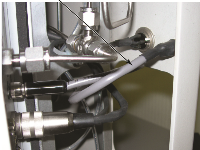
Figure 4: Internal view detail: 12V grey power cable
