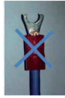
Terminal has been cut.
